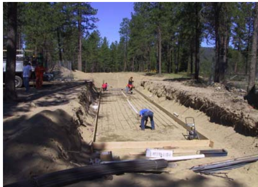
Workers prepare the ground and build forms for the truck weight scales at the Spokane Tribe's solid waste transfer station near Wellpinit, Washington.
